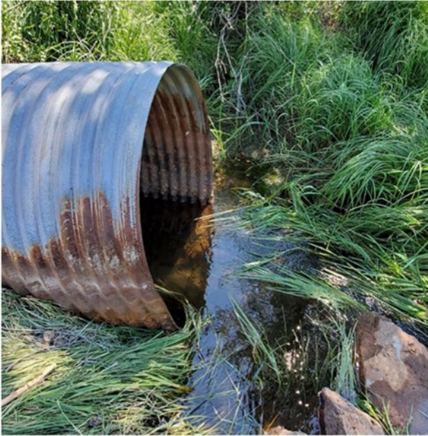
Photo #1. BEFORE (existing culvert barrier to fish passage)
